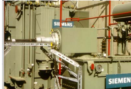
Figure 7: High-Voltage cable termination: Transformer - Petersen coil / Transformer Siemens / PCK Schwedt.
