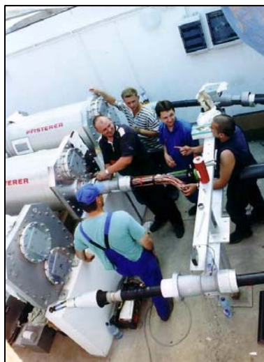
Figure 10: Cable installation before plug-in operation to the T-branching joint at Betchatow (Poland).
