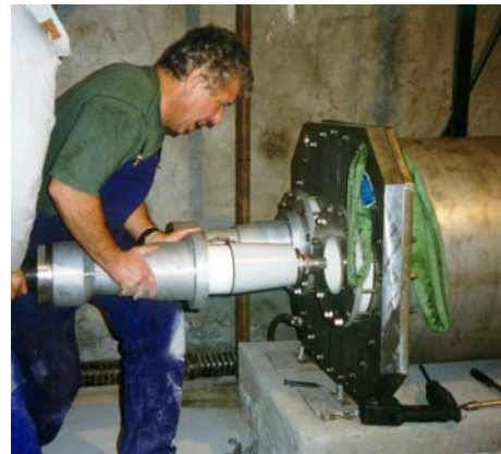
Figure 15: Plugging in the cable termination system to a T-Joint at BPSB Xian (China).
