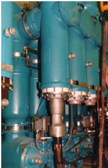
Figure 5: GIS Siemens Type 8DN9 with High-Voltage cable termination system and IEC extension adapter.
