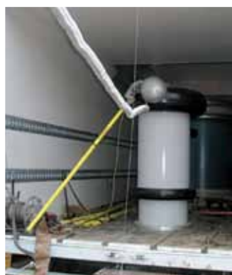
Reliable on site acceptance test
