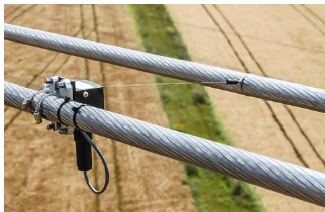
PT1 sensor for sub span oscillation measurement
