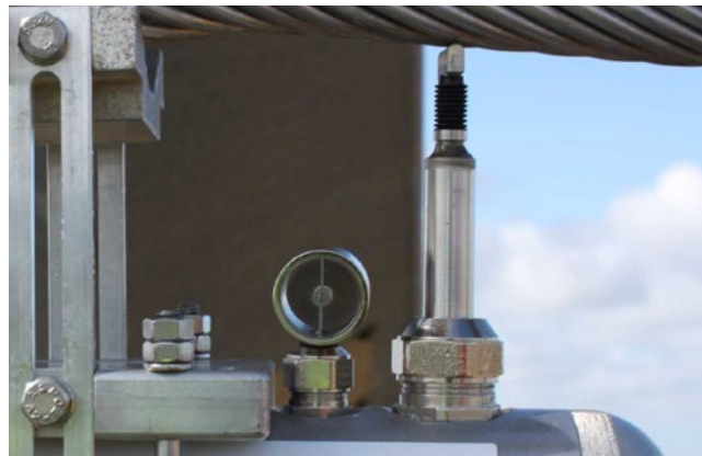
LVDT and wind sensor
